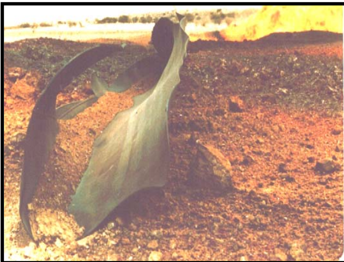
Rupture of a 20" Tape Coated Gas Pipeline.
